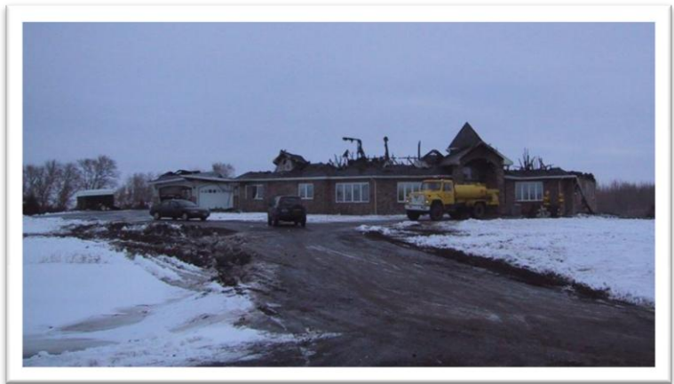
SIPs home damaged by fire
